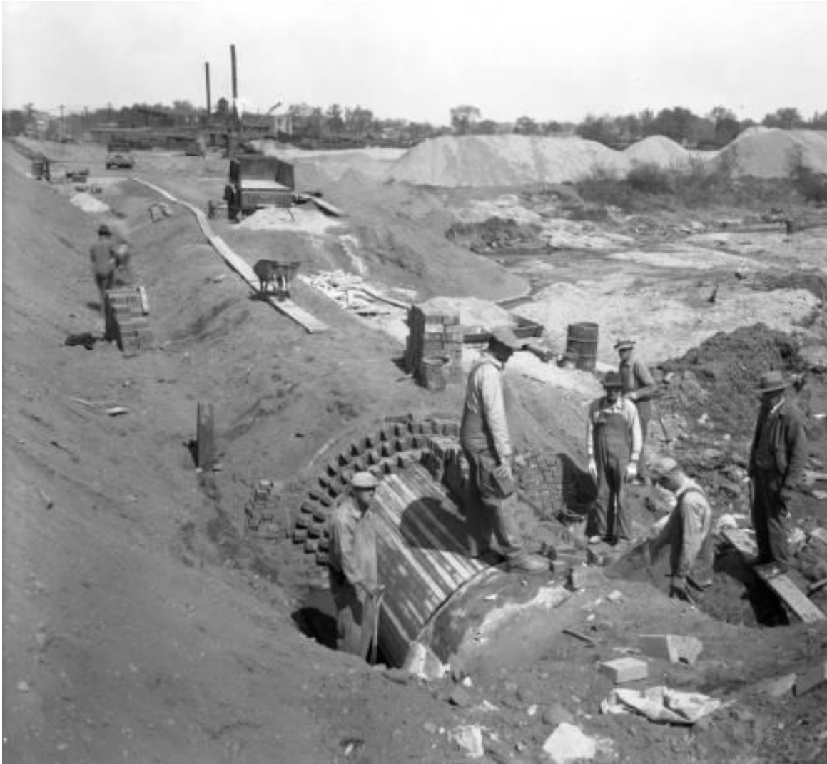
3-ring brick sewer line near South Platte River in Globeville. Circa 1930. Photo Courtesy of Denver Public Library, Western History Collection, Reference X-27588
