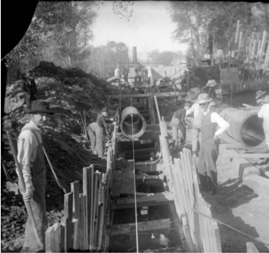
Men work with sections of sewer pipe and wooden forms. Circa 1909 Photo Courtesy of Denver Public Library, Western History Collection, Reference CHS-L1307
