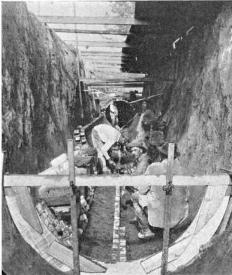
Building a 2-ring brick sewer line of the North Denver Sanitary Sewer. Circa 1910-1920. Photo Courtesy of Denver Public Library, Western History Collection, Reference X-29448
