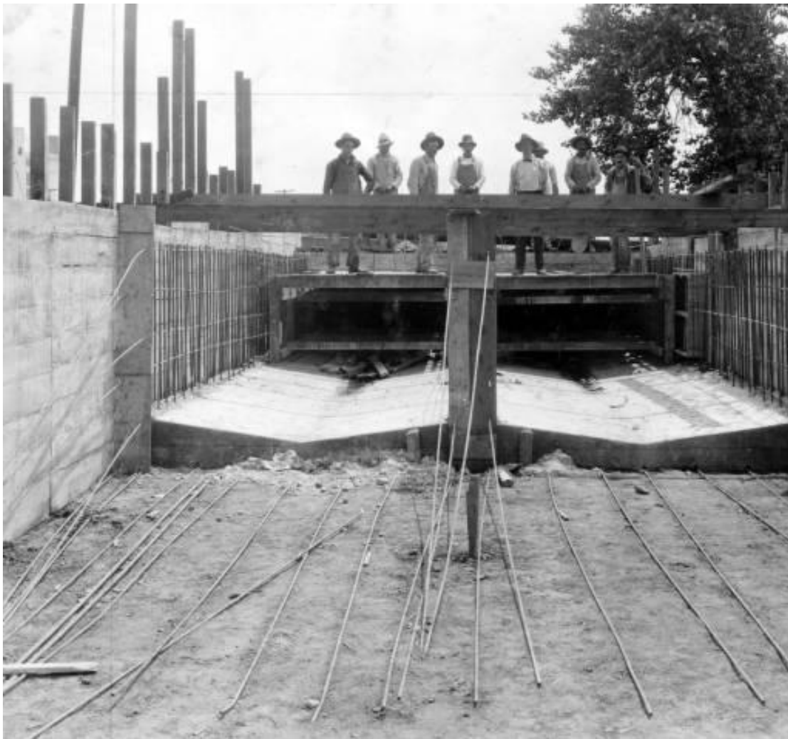
Outlet of the North Denver Storm Sewer, Circa 1910-1920. Photo Courtesy of Denver Public Library, Western History Collection, Reference X-29449
