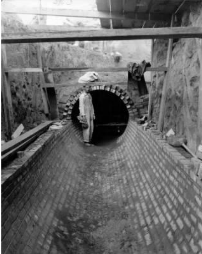
North Denver Sanitary Sewer, Circa 1910-1920. Photo Courtesy of Denver Public Library, Western History Collection, Reference X-29447
