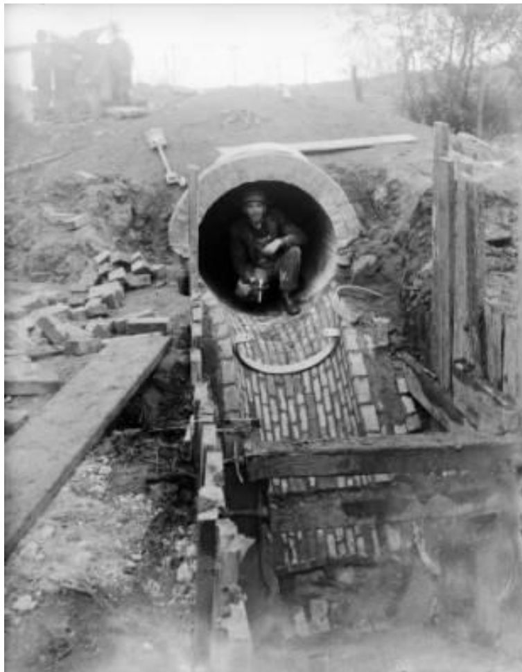
Workman in sewer outfall near South Platte River. Note the longitudinal pattern of the bricks in the sewer line. 1909. Photo Courtesy of Denver Public Library, Western History Collection, Reference CHS-L2696
